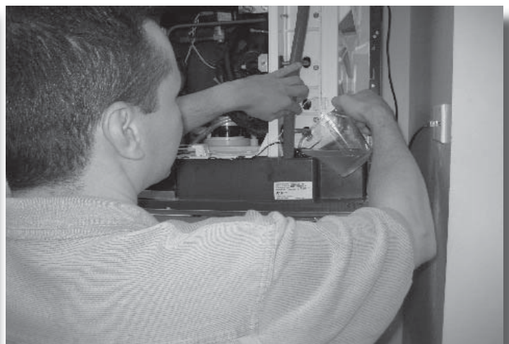
6. Wait until purge valve light goes out, then pour in scale remover.
